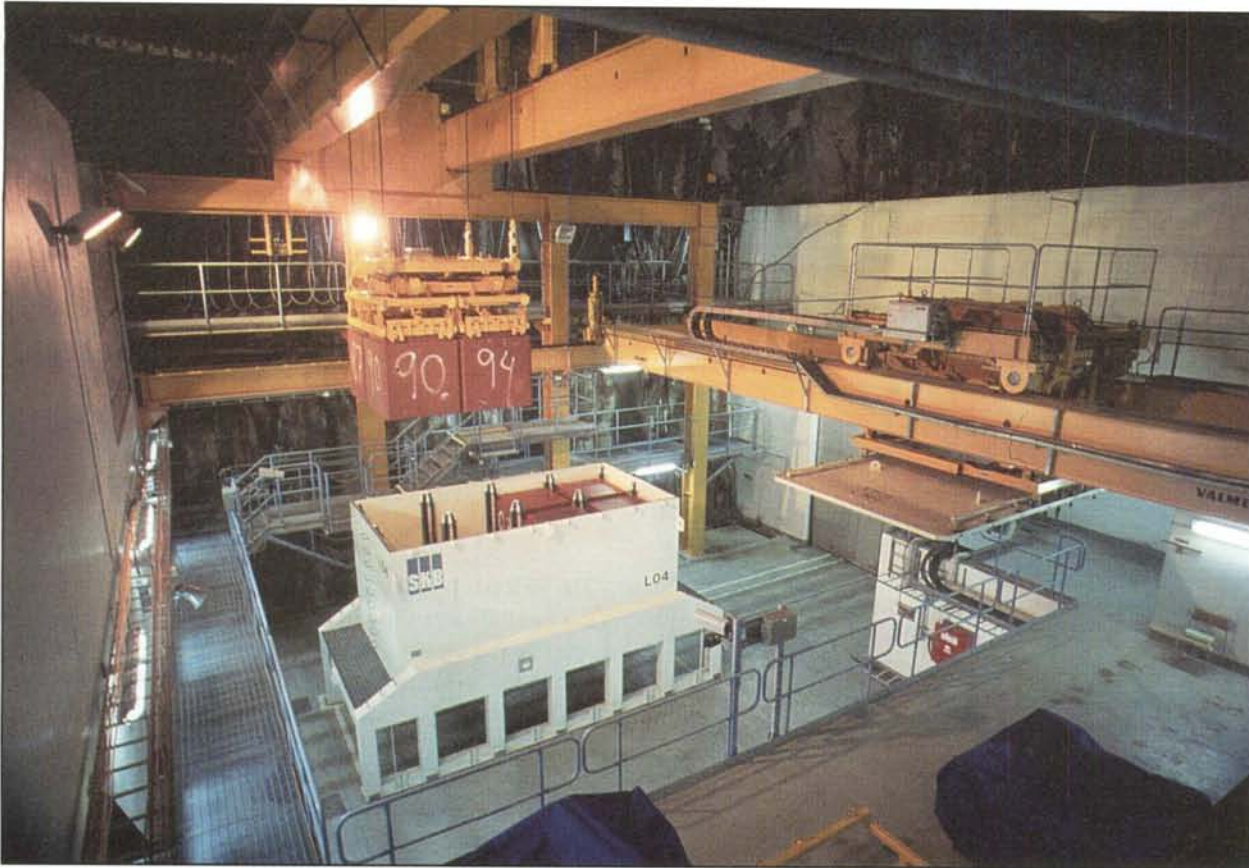
Figure 4-2. The operational waste is transported in special transport containers. In SFR the waste packages are unloaded with remote-controlled handling equipment.
