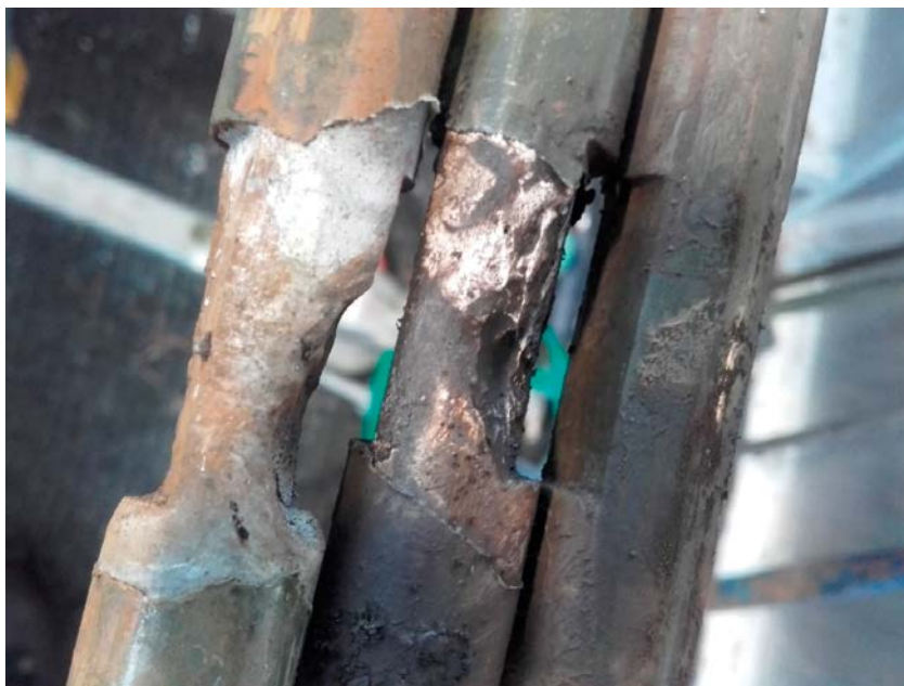
Figure 3-6. Corrosion attacks on rods from KFR102B.
