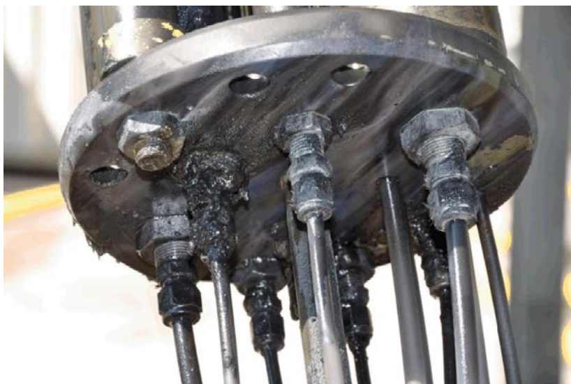
Figure 3-12. The bottom side of the lower holder for water level pipes (standpipes). Several of the connections were leaking when tested due to corrosion.
