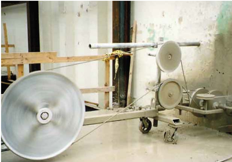
Figure A1-18. Typical Wire Saw drive in action cutting a section of wall.
