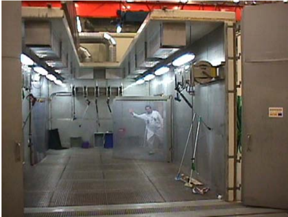
Figure 3-8. High pressure water decontamination facility at Oskarshamn.
